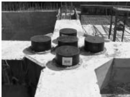
Fig. 7. Example of installation of five rubber bearings under one of the columns of the 10-story building in "Our Yard" complex
